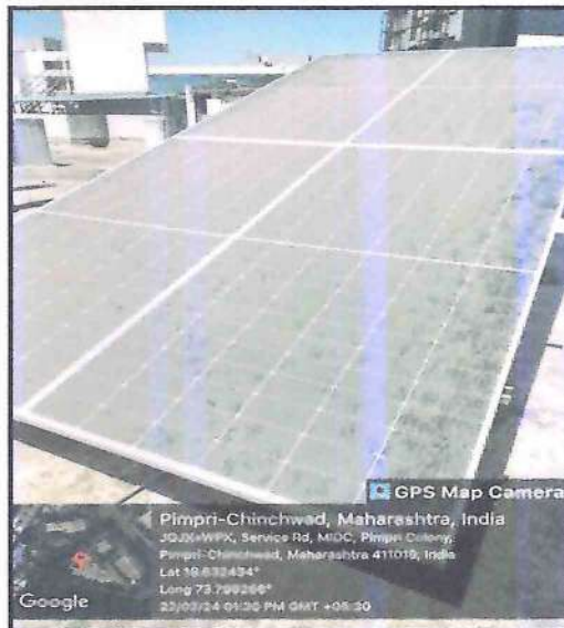
Photograph of Roof Top Solar PV Plant:
